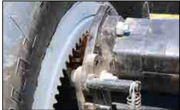
Fig 110 - Bin fill conveyor drive gears
