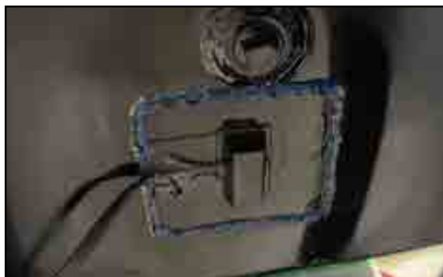
Fig 28 - Oil reservoir heater
